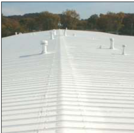
SOLAR REFLECTIVE COATING (S.R. COATING)
